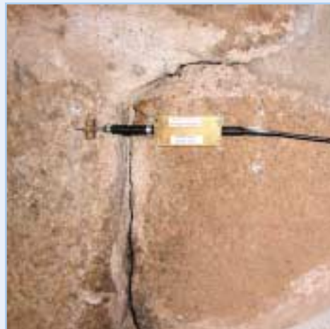
Extensometer as a fissure monitor.
