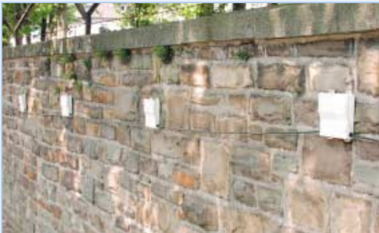
Wired X-Trigger along an extended brickwork structure.
