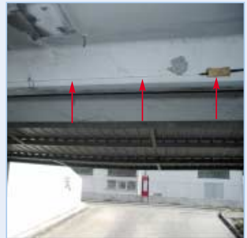
Optical Strand on a concrete beam.
